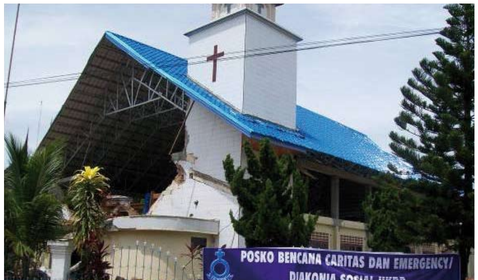
This church building suffered such serious structural damage in the earthquake that it will have to be rebuilt from ground level. Other church buildings have also been damaged or destroyed, as well as many Christian homes
