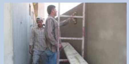
Plastering the walls of an apartment block for Iraqi Christians displaced within their homeland by anti-Christian violence
