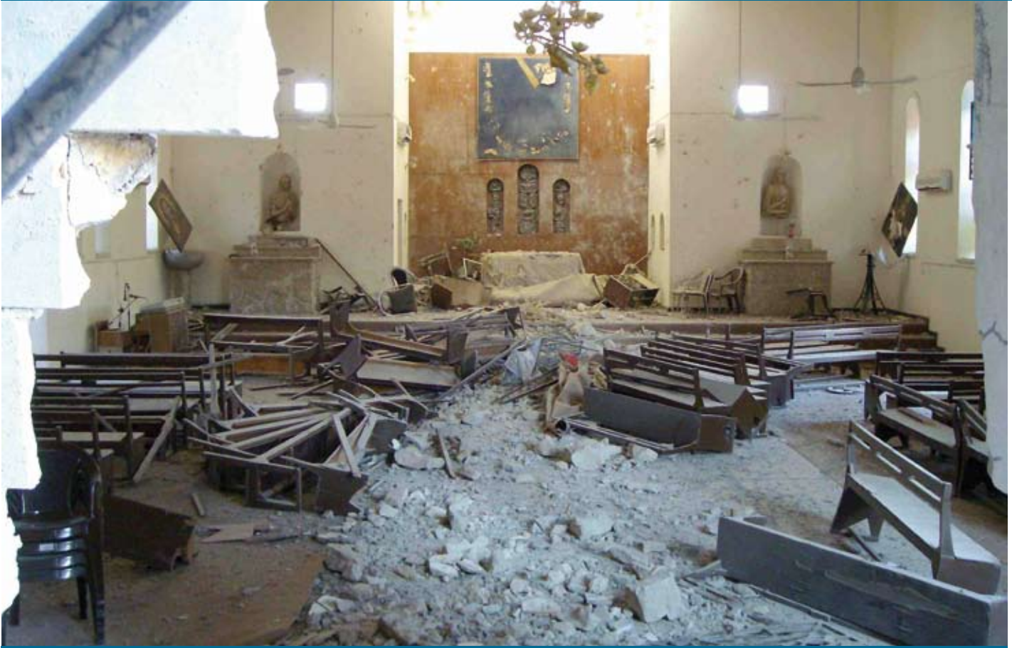
This church in Mosul, Iraq was severely damaged by a bomb on 26 November 2009
