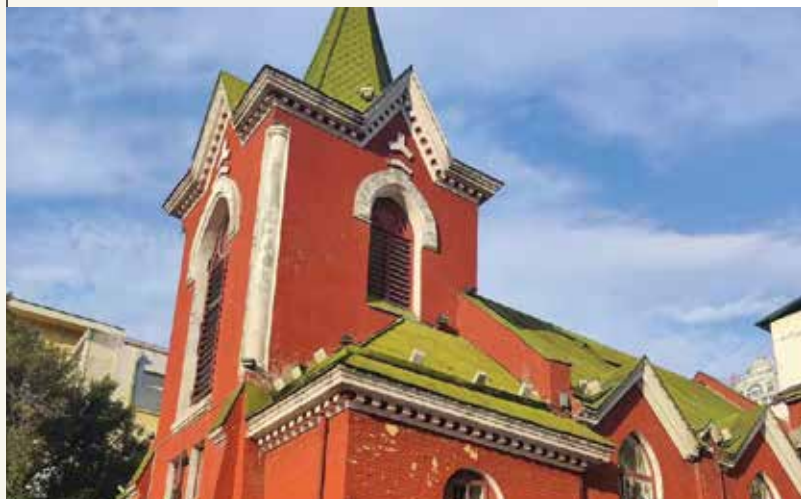
A church building in Harbin, Heilongjiang Province. The church was closed in 1967 during the Cultural Revolution, and only re-opened for worship in 1980
