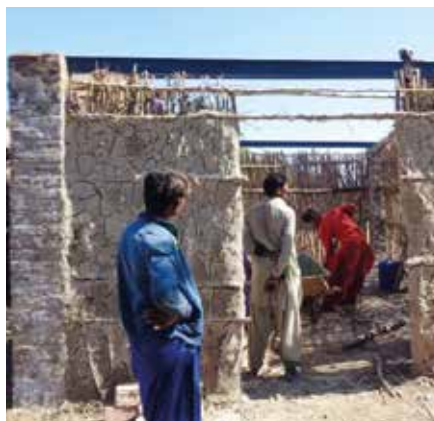
One of the new Barnabas-funded homes under construction, showing the brick-built pillars supporting the mud walls. Some of the iron girders that will support the mud roof are in place
