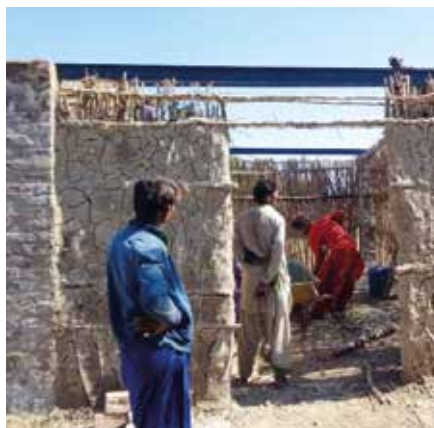
One of the new Barnabas-funded homes under construction, showing the brick-built pillars supporting the mud walls. Some of the iron girders that will support the mud roof are in place
